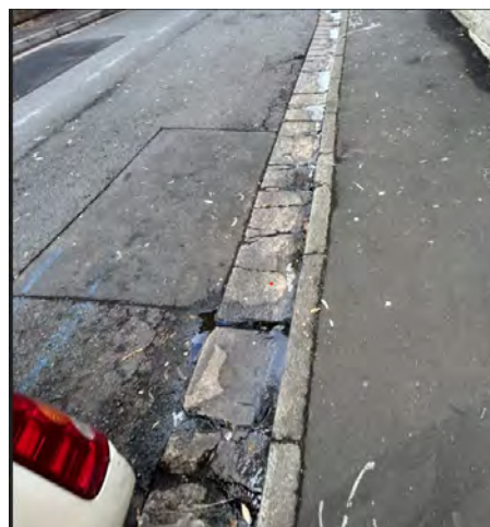
Condition 5 – Very poor
