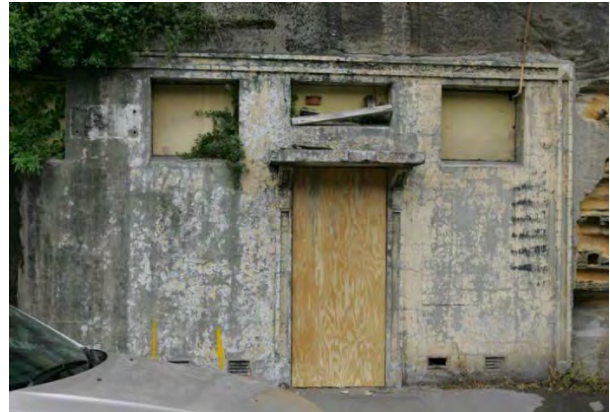
Condition 5 (very poor)
