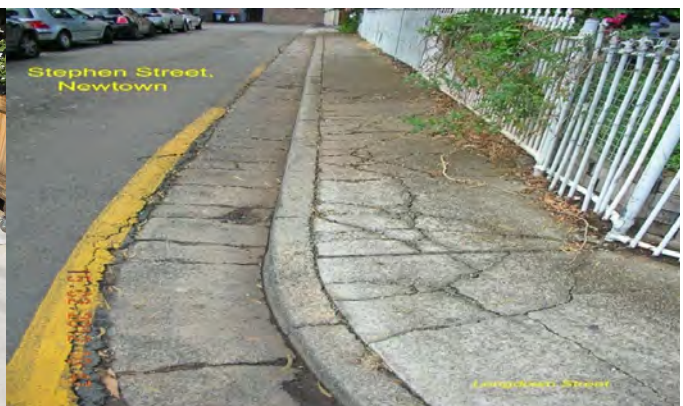
Condition 5 – Very poor
